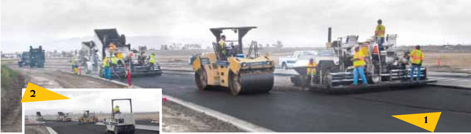
(1) Paving Crew Installing first 3 inch lift of AC on Tustin Ranch Road.
