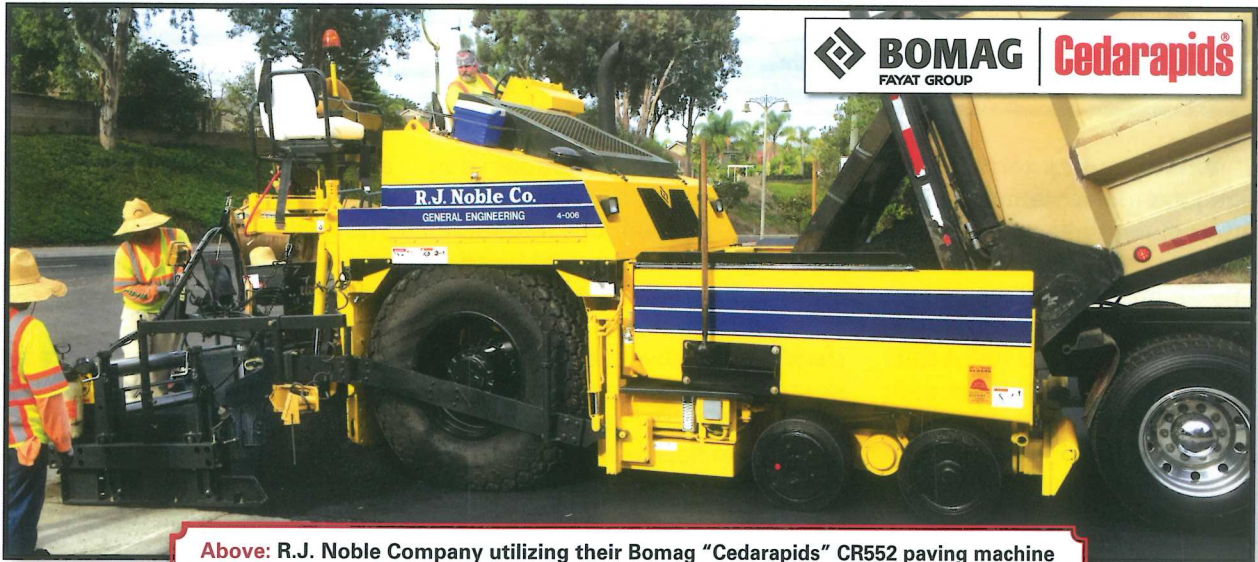
Above: R.J. Noble Company utilizing their Bomag "Cedarapids" CR552 paving machine on a public works street project in Mission Viejo.
